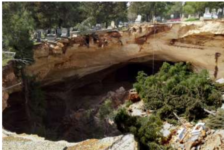
Figure 10. Collapse of the new cemetery in Gaziantep (phot. A. Yamaç)
